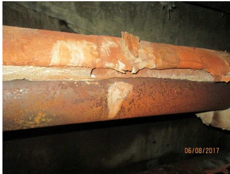
Typical pipe corrosion observed.
