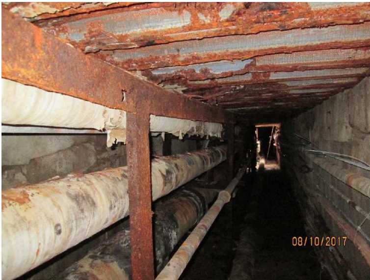
Corroded form deck and widened horizontal crack on right wall in main tunnel.
