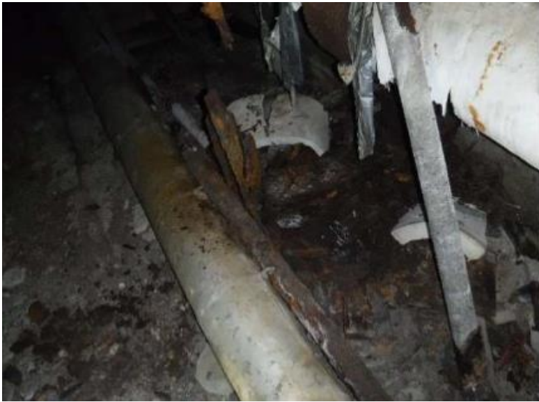
Failed pipe support base.
