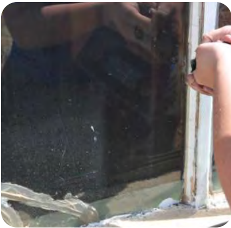
1. Remove all broken glass
