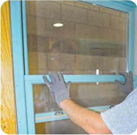
7. Ensure window is operational
